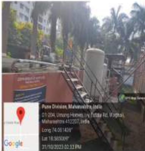
Sewage Treatment Plant
